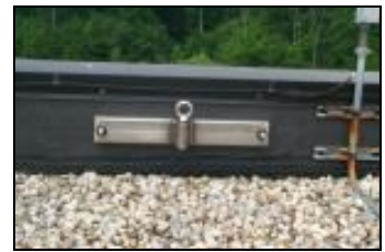
Roof Mounted Anchor Point
